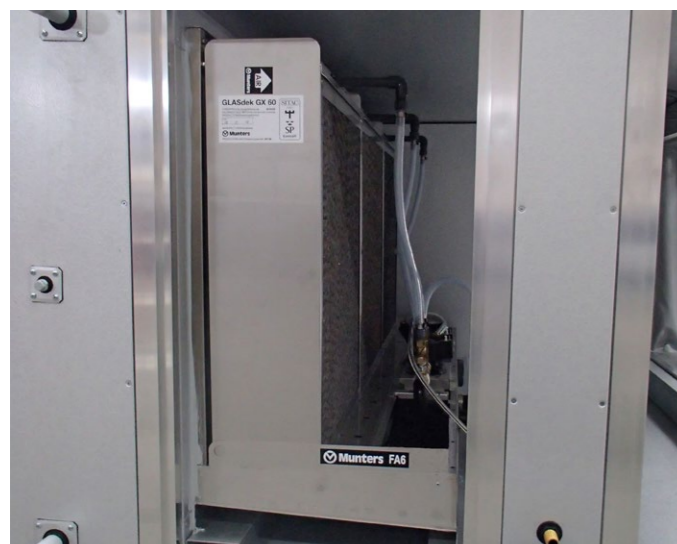
Example of an FA6 installation in a section of an airhandling unit
