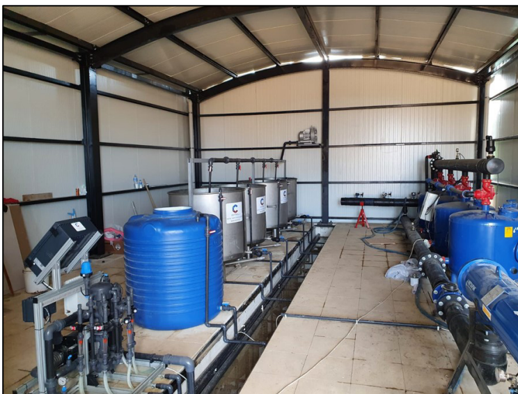
Figure 1: Green JET Unit, Installed and Running
