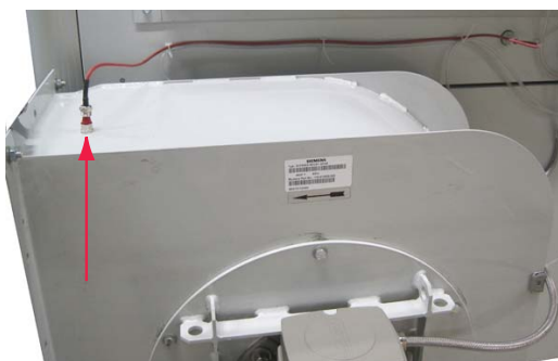
Figure 3.21 PT1000 connection at reactivation fan
